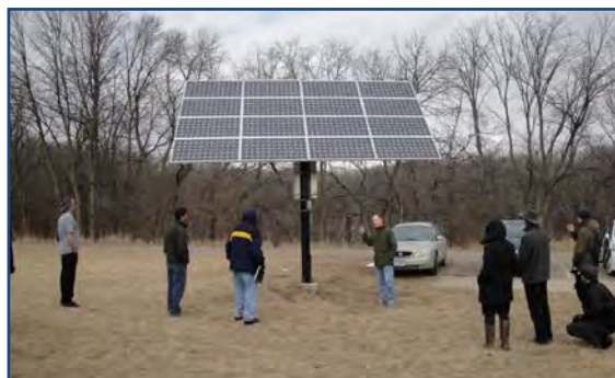
Ground Mount System, CERTs
