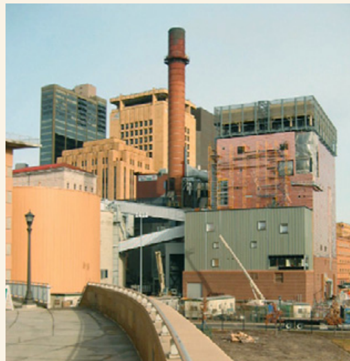
In January 2003, construction is almost completed at the new combined heat and power plant in Saint Paul
