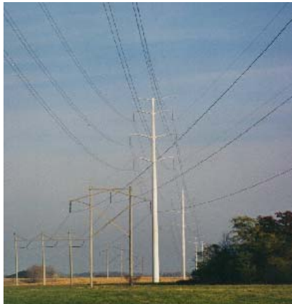
High Voltage Transmission Lines
