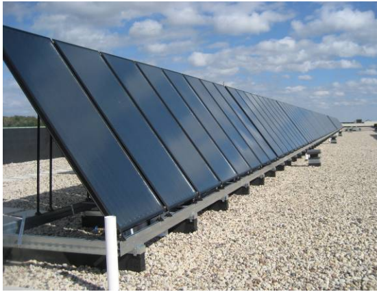
Minnesota-made solar thermal hot water panels
