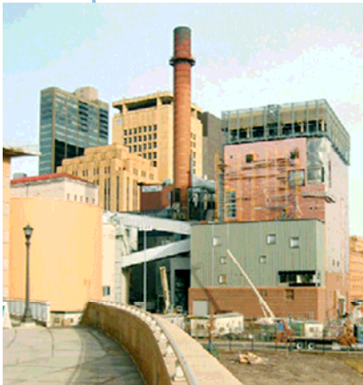
In January 2003, construction is almost completed at the new combined heat and power plant in St. Paul
