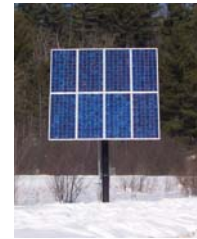
Tracker pole PV system
