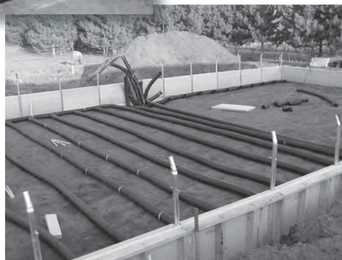
Figure 2. The second layer of tile line. The tile line was hooked up to the solar panels in the center of the picture.
