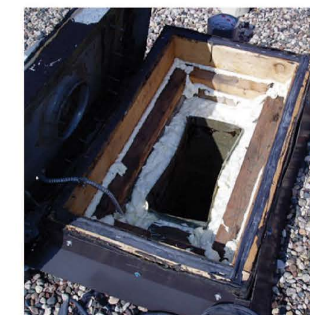
Seal leakage below fans at curb
