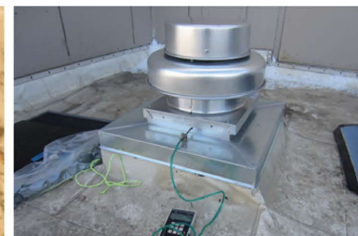
Replace with ECM fans
