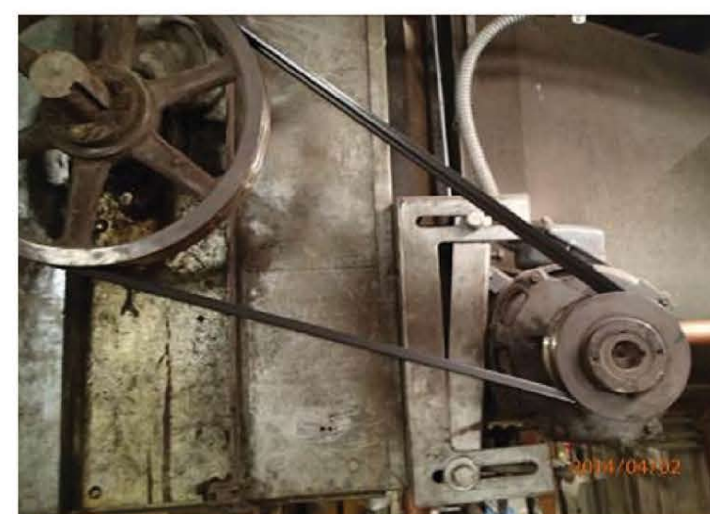
Re-sheave (change pulley size) to reduce fan speed
