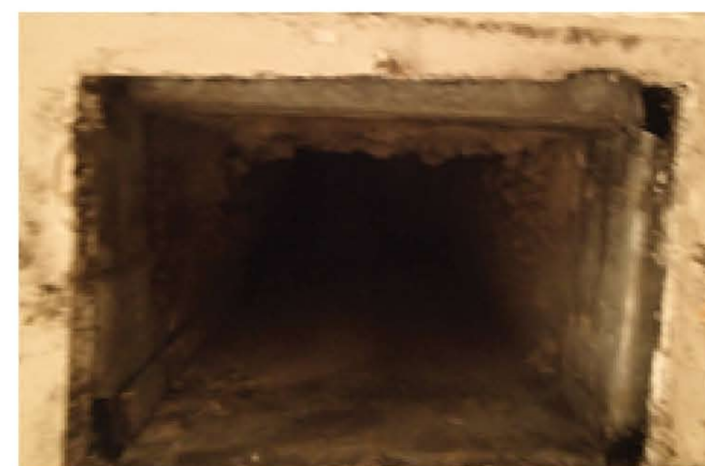
Seal duct leakage at inlet
