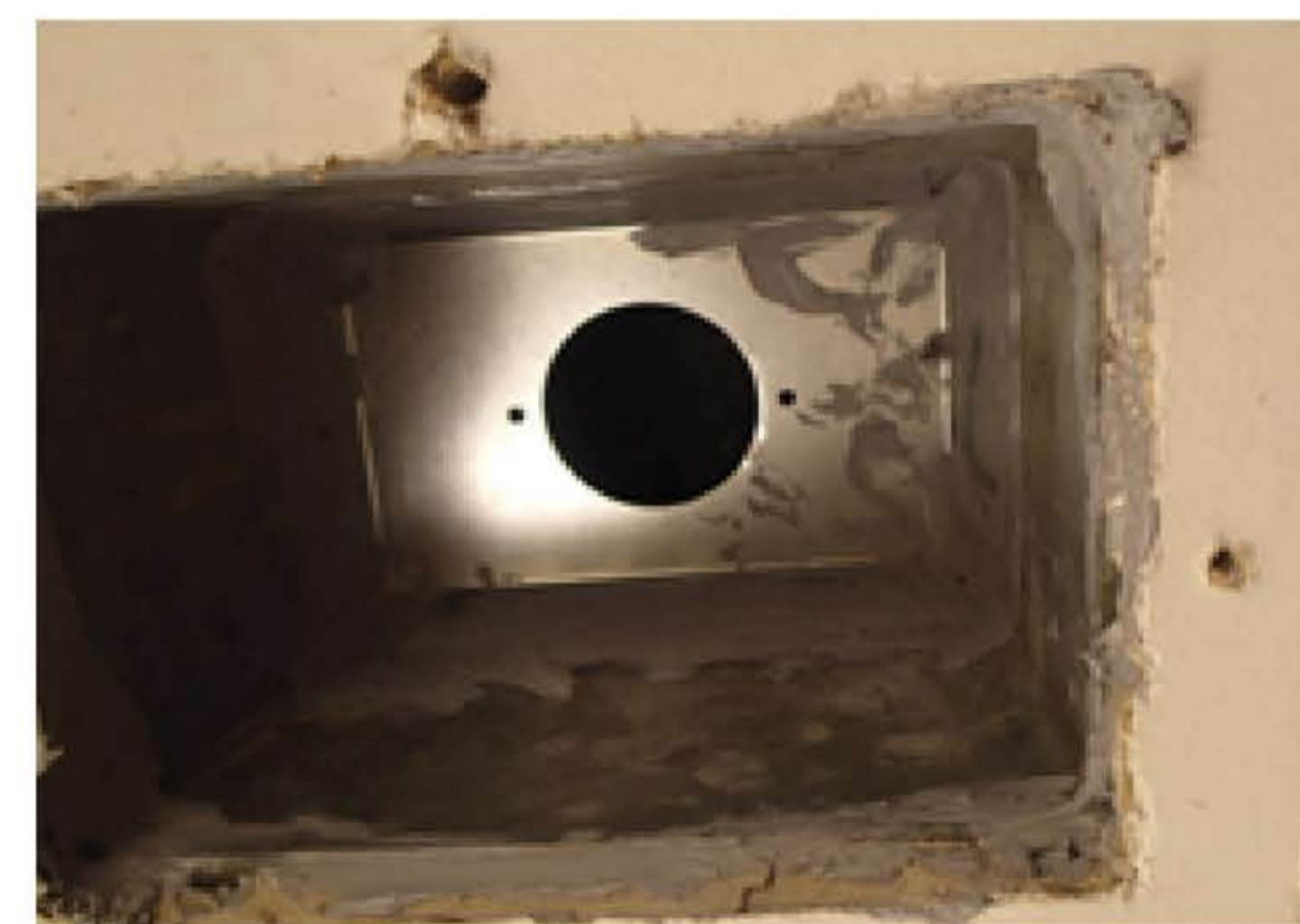
Balancing devices prone to clogging - replace with fixed orifices
